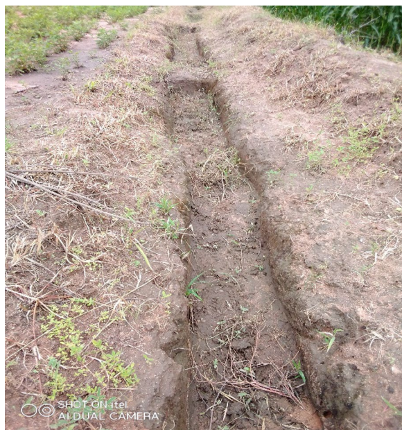
Fig. 5 STDC ridges reinforced with variants of infiltration pits in Marange with dimensions of 5 \times 0.5 \times 0.5 m for Length x Width x Height. (Photos by George Nyamadzawo)
