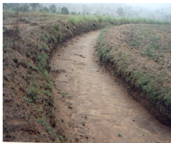
Fig. 3 The standard contour ridge, a channel which is meant to dispose excess water from the field
